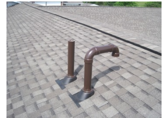
Painted Vent Stacks
