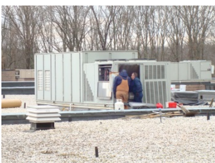
Problematic HVAC Unit
