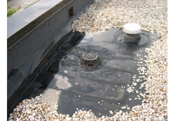
Improper EPDM Repairs
